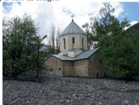
Figure 4 Yard of the Church of Mleta covered with debris flow mass and solid fractions
