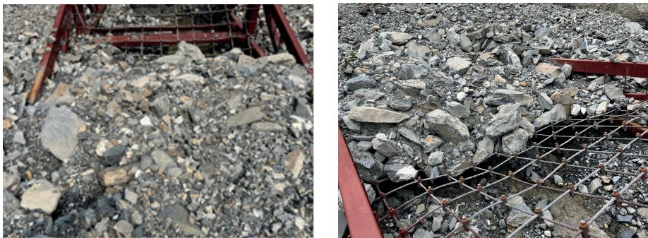
Figure 10. Debris Flow Regulation Elastic Barrage in the Mleta River Gorge (June, 2023)
