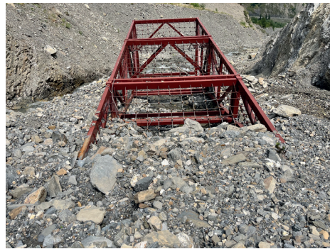
View of the structure after the debris flow passage
